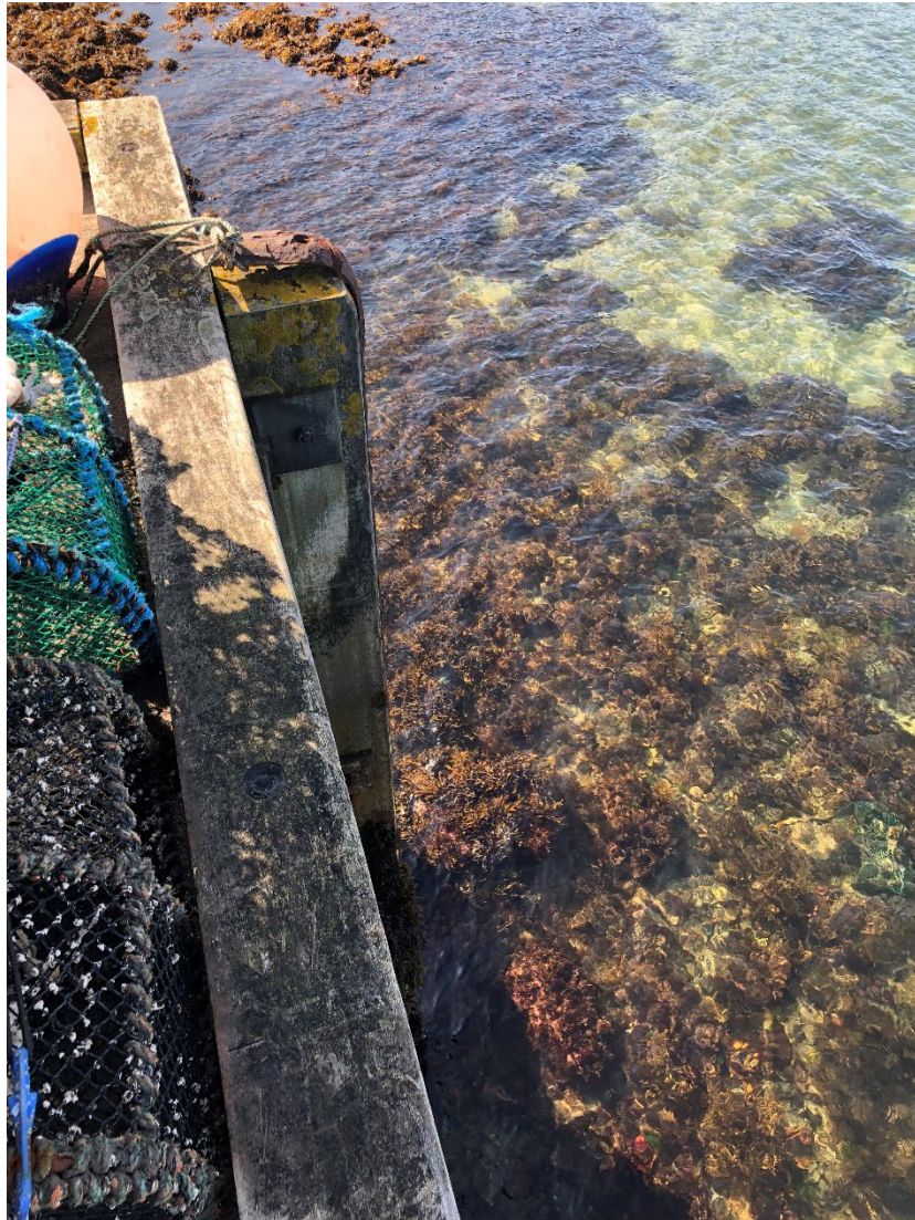
Image B7. Bunessan, wooden fendering in disrepair
