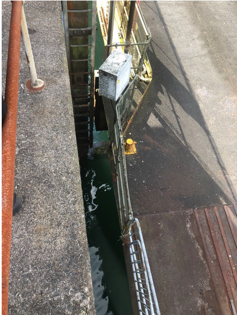
Image B1. Craignure, ladder does not extend below waterline
