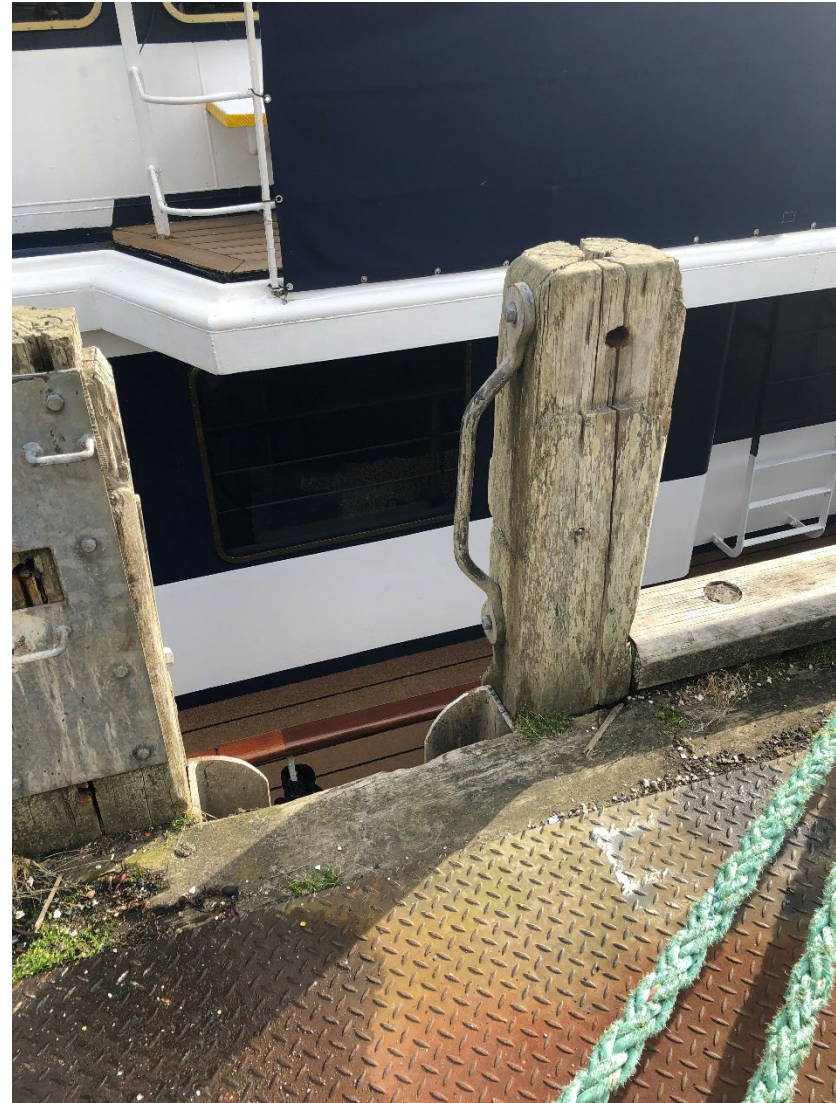
Image B2. Craignure, ladder with missing handrails or grab loops
